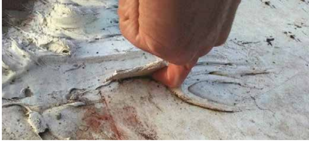
Poorly sealed flashing at PV standoff
